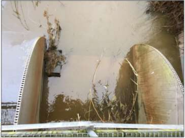
Figure 1.6. Photo of tilting weir (in lowered position) from above. Elver pass can be seen on the left hand side.
