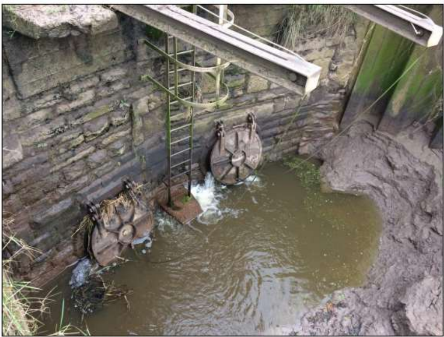
Figure 1.4. Photo (taken during low tide) of tidal flaps controlling ingress of water from the River Severn to the Low Level Carrier (left hand side) and High Level Carrier (right hand side).
